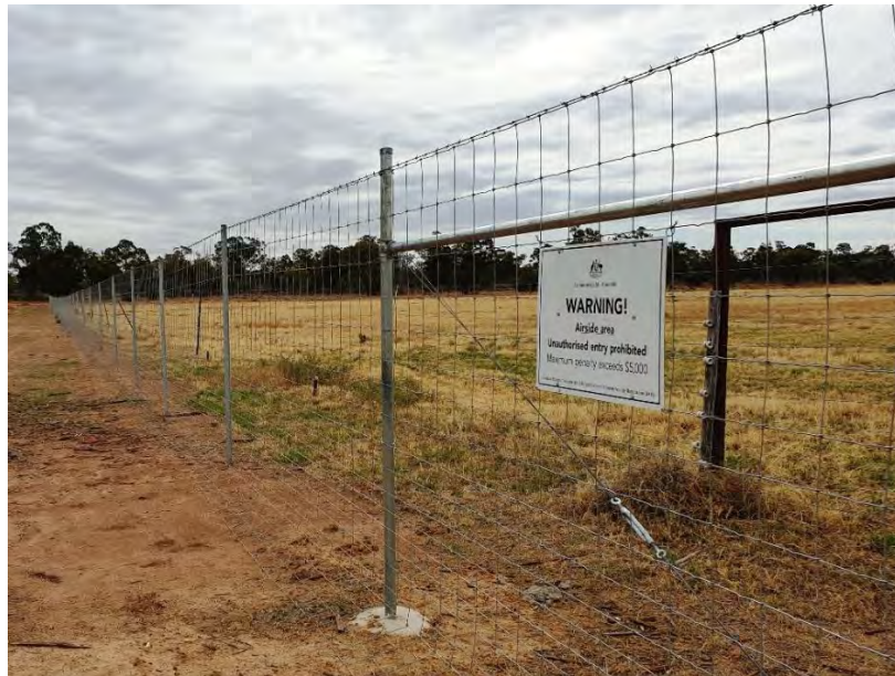
Figure 3: Example of animal exclusion fencing at Aerodromes
